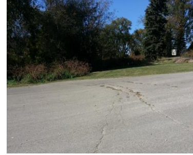
Sloughing at Lincoln Drive Park boat ramp
