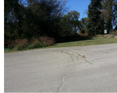
Sloughing at Lincoln Drive Park boat ramp
